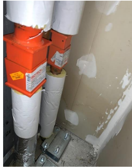
Figure 2: Newly installed and designed expansion compensators with guides.
