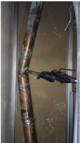
Figure 3: Bowed/bent piping due to failed expansion and support system
